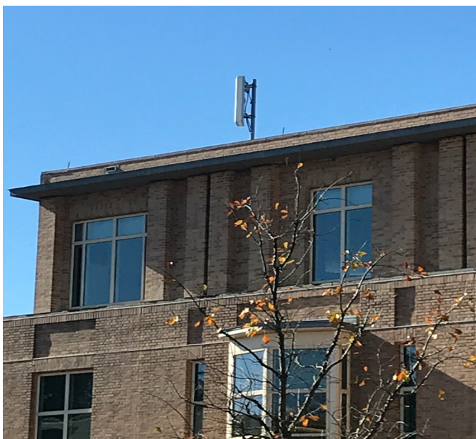
Figure 5-2: One node of an outdoor DAS installation near a sports venue
