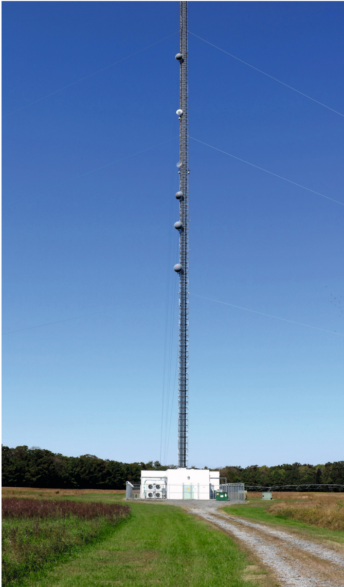
A week after the project started, WBOC was on-air and signal strength increased approximately 20-fold.
