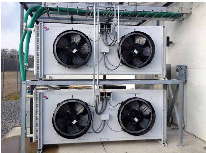
The concrete pad outside the broadcast facility had to accommodate two exchangers because it was decided to keep the old transmitter in service.
