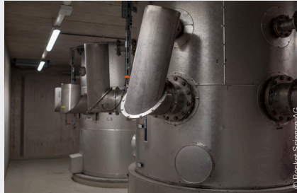
The chimneys waste incineration plant.
